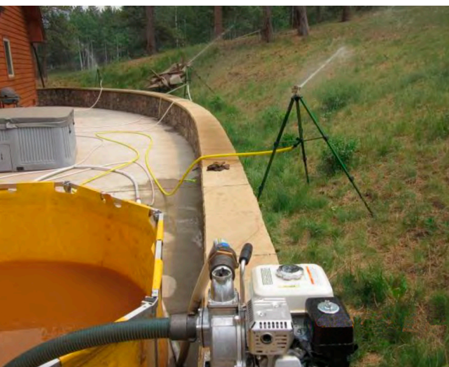
Firefighters hired by Chubb set up a sprinkler system to help protect the Ward home.
